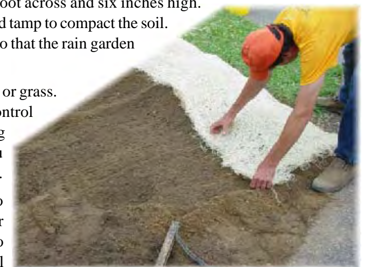
Erosion control matting made of coconut fiber is carefully placed along the berm to prevent erosion on the downhill side of the rain garden.
